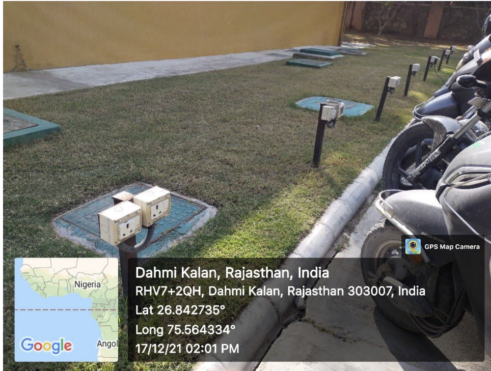
Picture 8: EV charging points .
